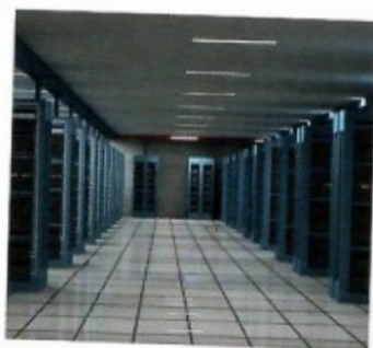
5 Digital switching equipment
